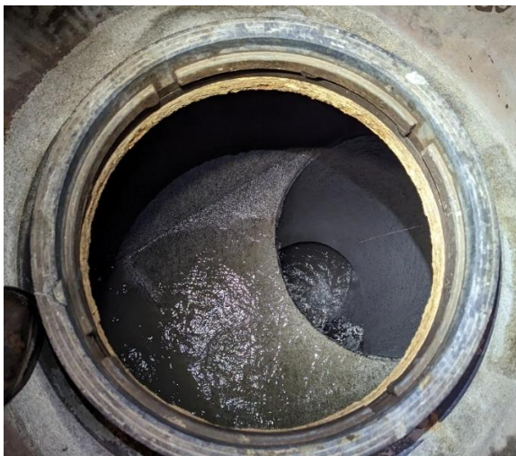
Figure 1: Manhole opening offset from interceptor
